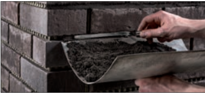
The grouting with a pointing trowel and a metal float in the horizontal direction.
